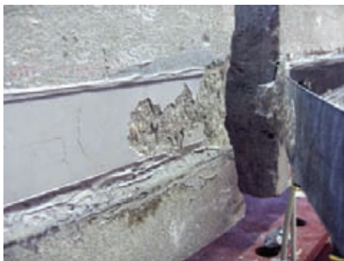
Figure 20. Debonded laminate after failure
