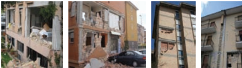
Figure 10. Overturning of masonry infill walls – l’Aquila 2009.
