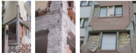
Figure 9. Damaged beam-column joints-Overturning of masonry panels – l’Aquila 2009.
