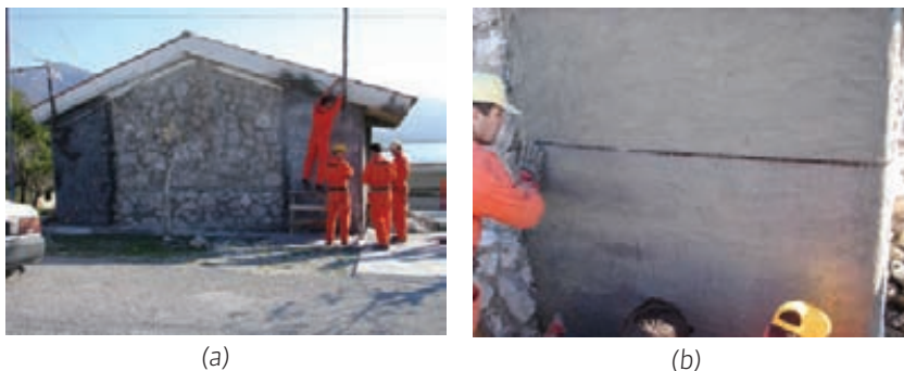
Fig. 9 Pilot application of the TRM strengthening technique: (a) Masonry building; (b) TRM layers are applied “as usual” using trowels.
