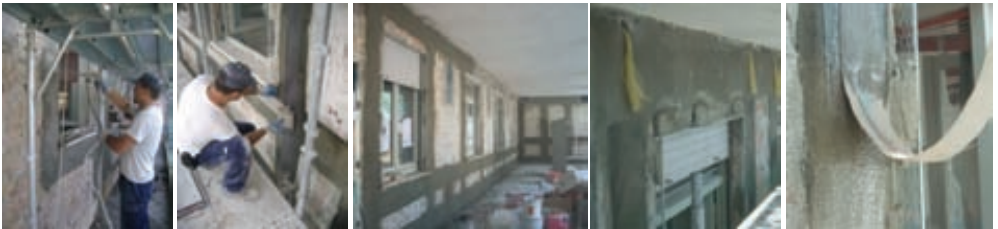
Figure 19. Strengthening of the external masonry panels using flax fiber sheets and aramid fiber connectors.
