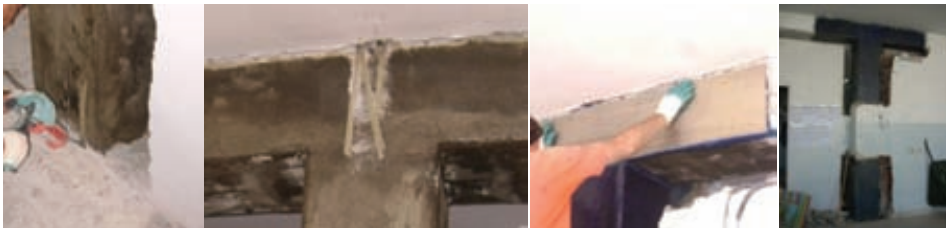
Figure 18. Damaged columns-Steel fiber connectors and strengthening phases.
