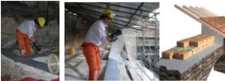
Figure 4. Strengthening of the ring corbel masonry beam with FID-Steel Hardwire® impregnated with epoxy.
